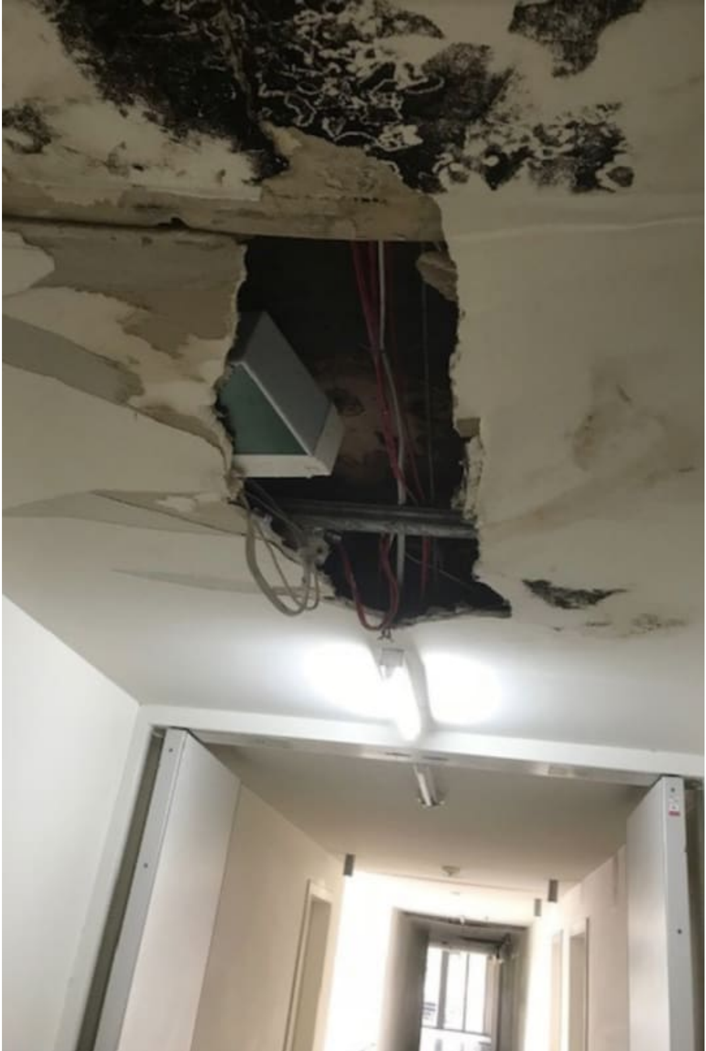
Damage to property at 19 Gadigal Avenue, Zetland. Supplied
